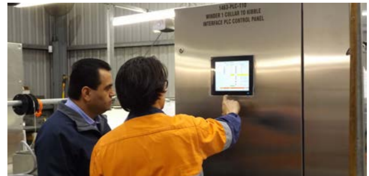
CERBERUS Factory acceptance testing with Hahn Electrical ( Rio Tinto Mongolia Project)
